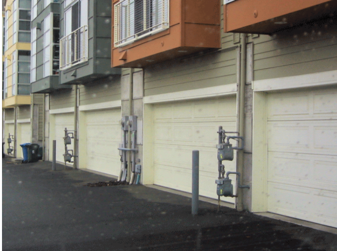
Figure 18.120.020.F.2.b. Place utility meters in less visible locations. Note that this example is acceptable on a service alley but not near a street or residential walkway.
