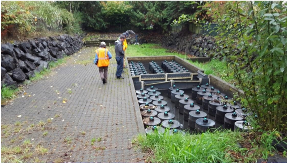
Figure 3 - Stormwater Filtration at the City of Olympia's Giles Avenue Facility
