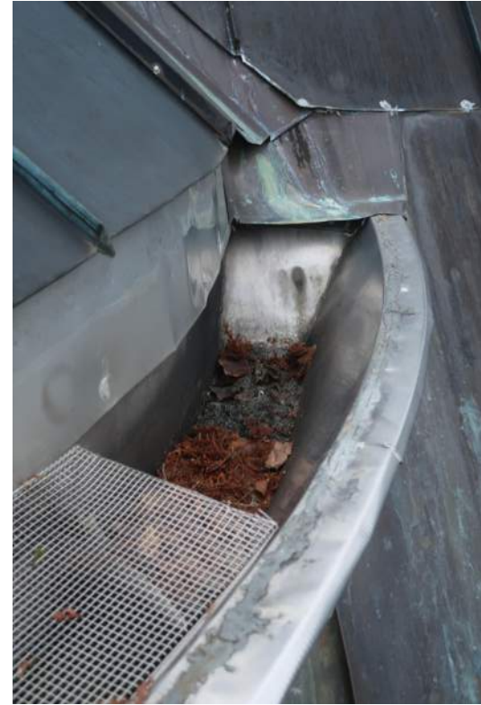
8 S.S. GUTTER AND PARTIAL DEBRIS SCREEN
