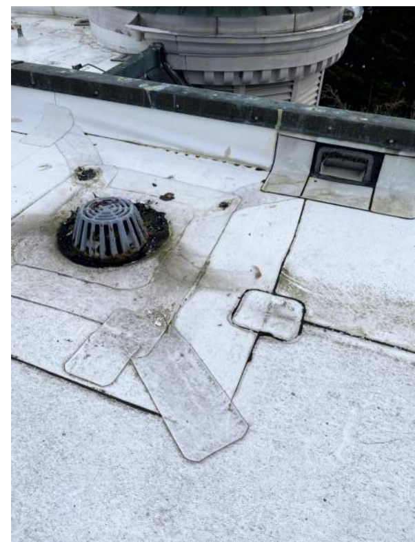
14 ROOF DRAIN AND METAL SCUPPER ON BUILDING 'B' LOW-SLOPE ROOF
