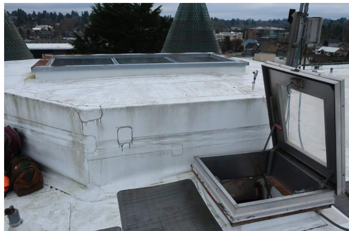
11 ROOF HATCH AND RAISED MECHANICAL VENT
