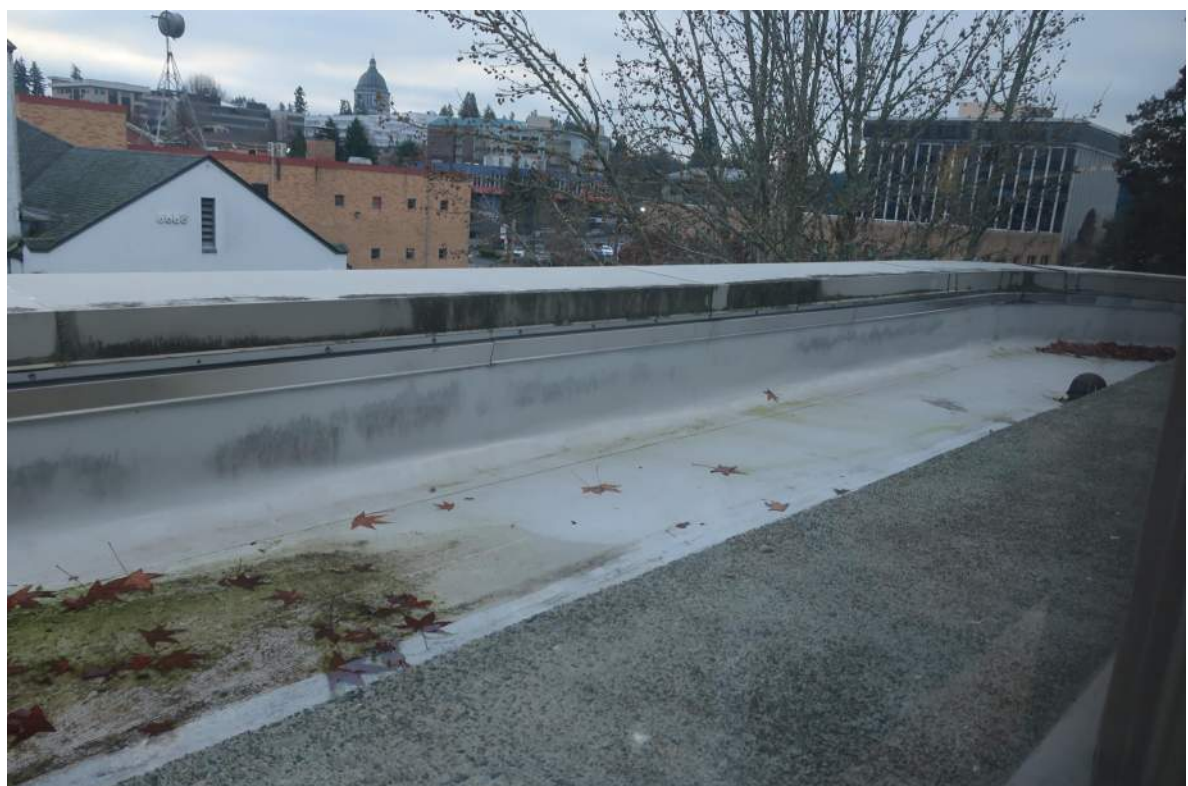
16 BALCONY B1 ROOF WITH LOW-SLOPE ROOF, METAL TERM BAR, AND METAL COPING
