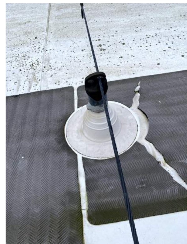
13 ROOF ANCHOR ON BUILDING 'B' LOW-SLOPE ROOF
