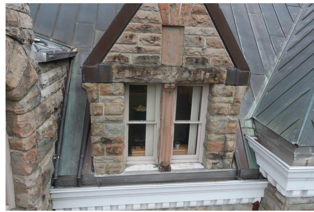
4 SOUTHWEST DORMER WITH S.S. INTEGRAL GUTTER AND APRON FLASHING, PTD METAL CORNICE, AND RAKE FLASHING
