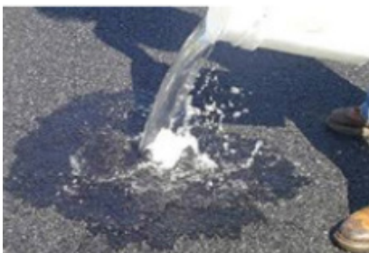
Increased erosion and sedimentation prevention is needed for permeable paving to prevent plugging and reduction of infiltration (Element 14).
