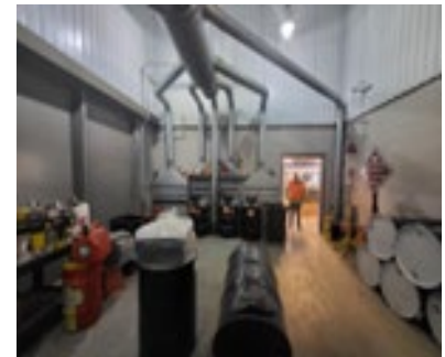
Figure 4-2. HazoHouse Bulking Area
