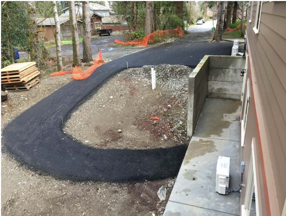
Bike path from above, flat asphalt pad to sidewalk and on turn around, and and View of Murihead behind trees with orange fences and also in upper right corner.
