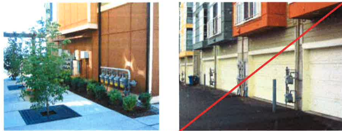
Good and bad utility meter configurations. The example on the left is consolidated and somewhat screened by landscaping elements, whereas the right example is exposed and degrades the character of this project.
