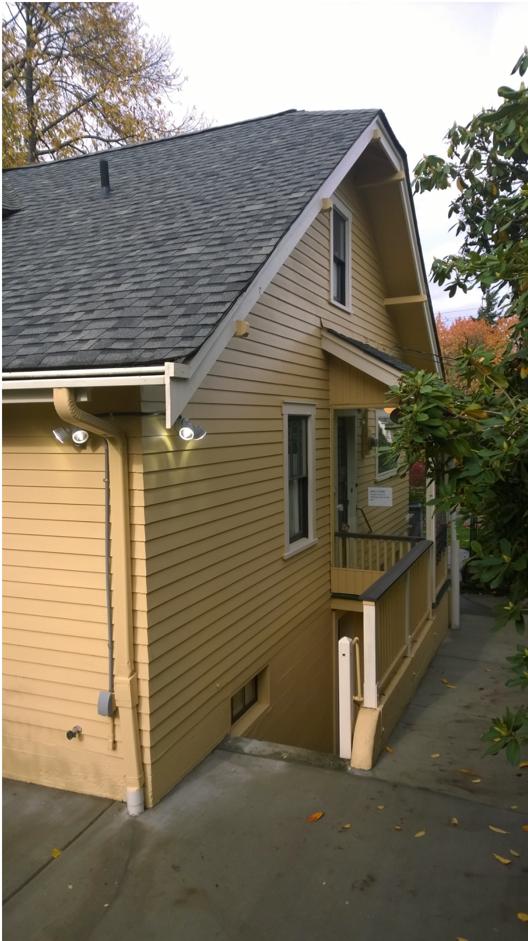
Figure 6: Side (East) Elevation. Significant drainage work involved new paving and safety railings were installed.
