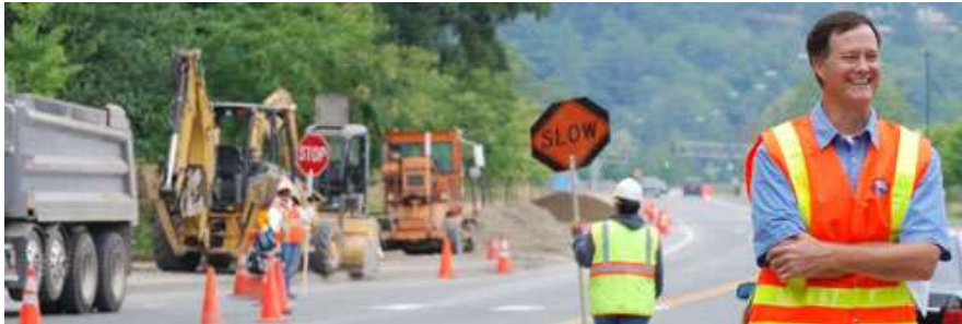
City project manager checks in on a capital facilities project.
