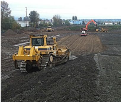
Minimizing site disturbance must be balanced with other criteria, including ADA accessibility, cut/fill balancing and parking lot slopes (Element 1).
