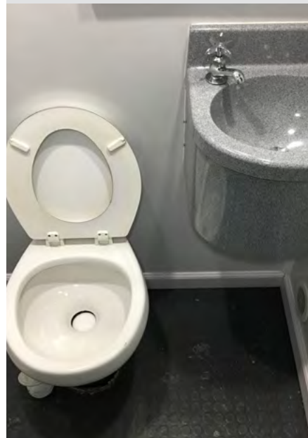
Flush toilets and running water provide a more hygienic and appealing experience than the dry portable units.
