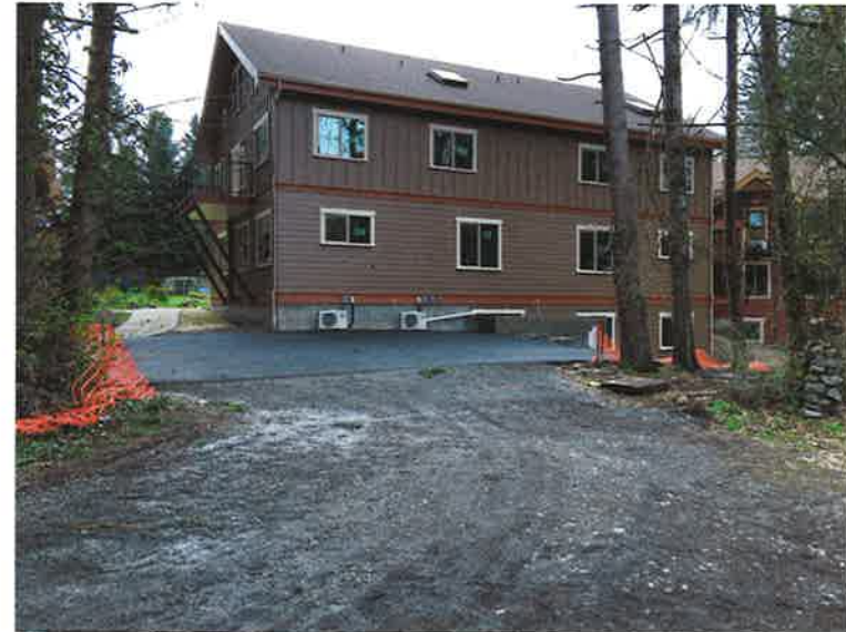
Asphalt pad in turnaround, connecting bike path to sidewalk, photo from Muirhead's west narrow part
