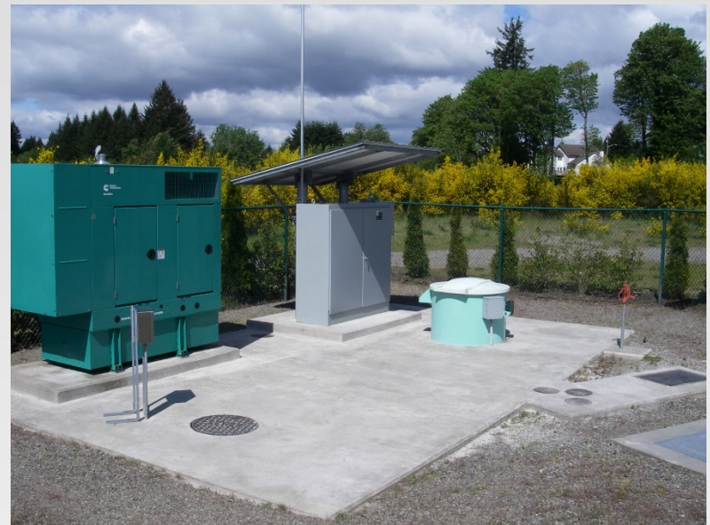
Briggs Village Lift Station
