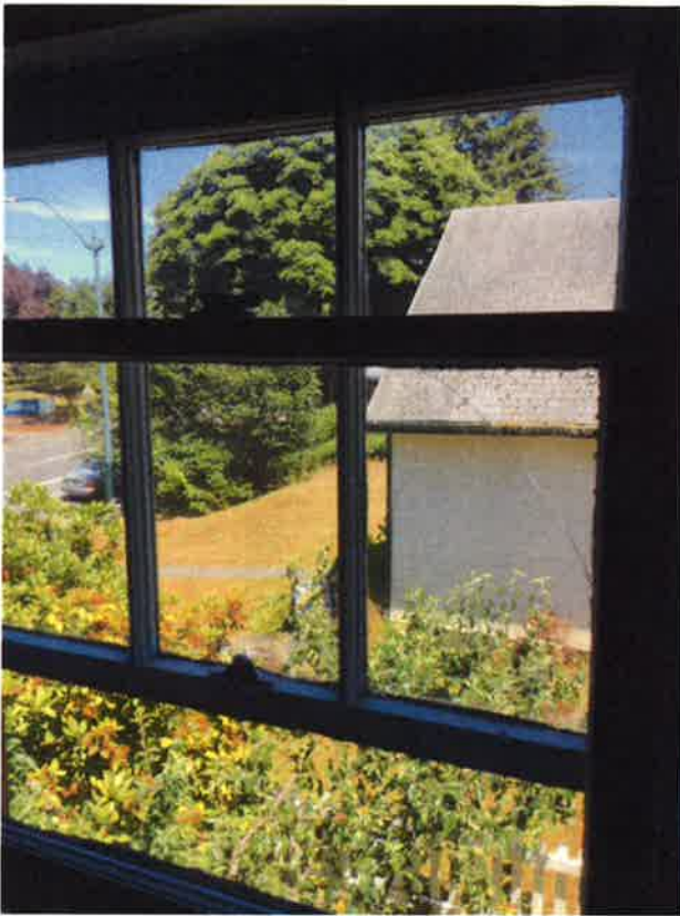
9 3rd floor hall broken window 2015
