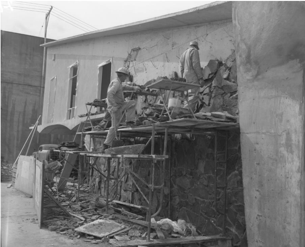
Capital Savings & Loan - construction photo – March 1963 Images Courtesy of WA State Archives – Parish Collection
