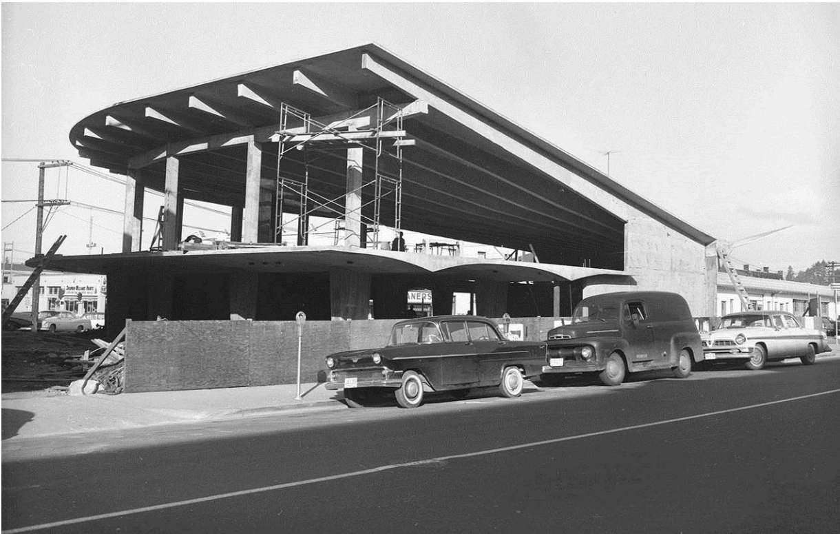
Capital Savings & Loan - construction photo – January 20, 1963 Images Courtesy of WA State Archives – Parish Collection
