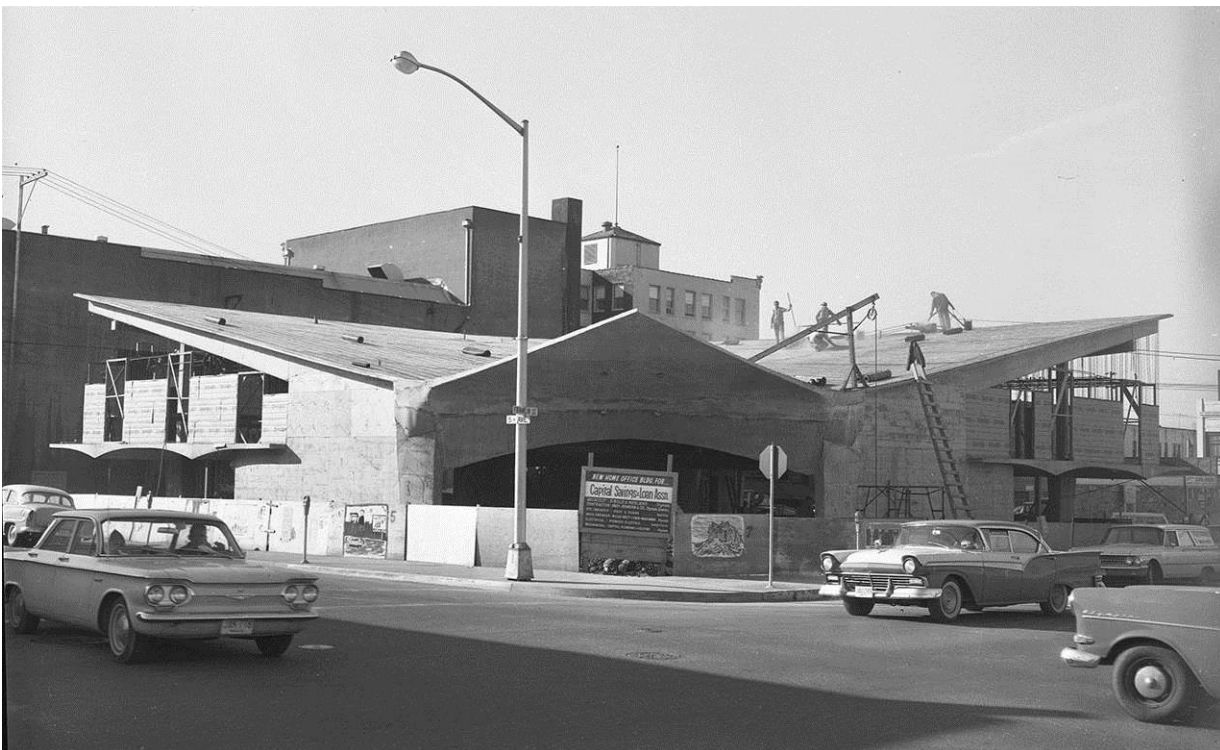
Capital Savings & Loan - construction photo – February 1963 Images Courtesy of WA State Archives – Parish Collection
