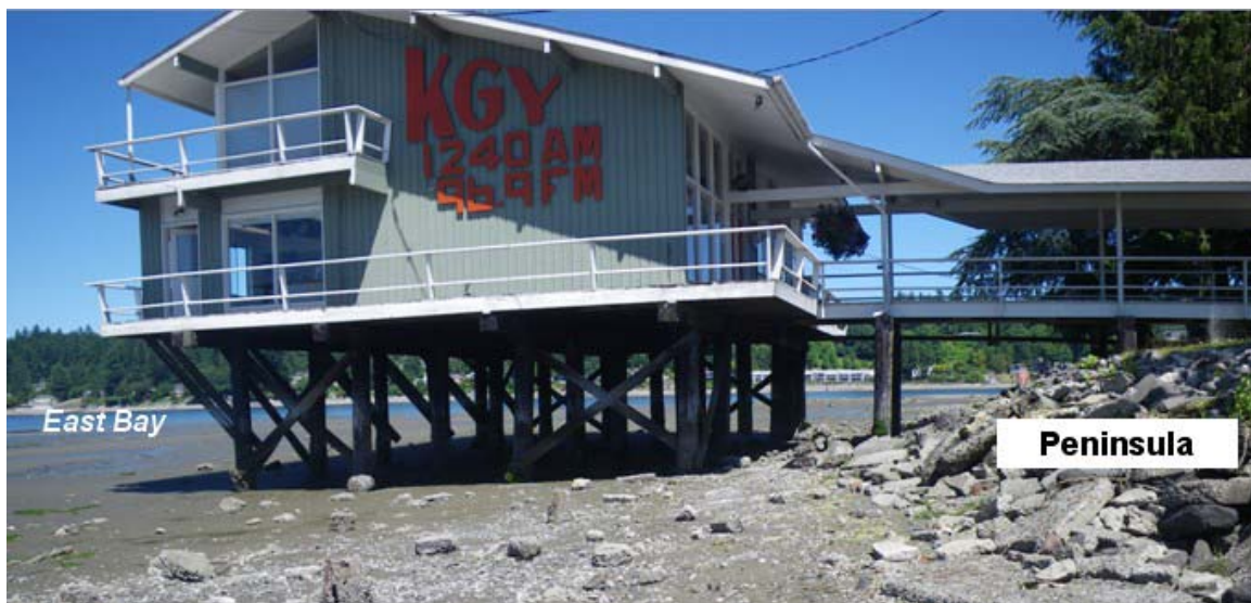
Figure 33. Overwater structure vulnerable to inundation and wave damage
