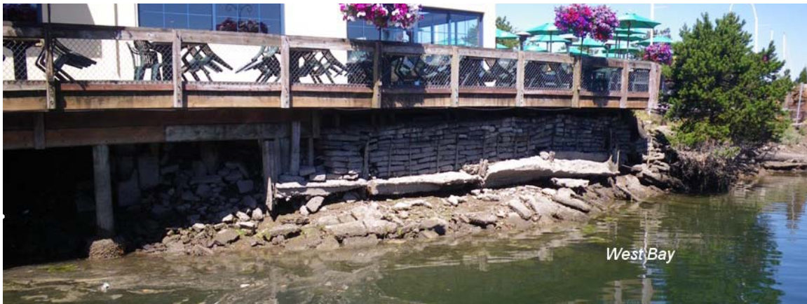
Figure 34. Exposed structural supports vulnerable to wave and debris impact at higher elevation
