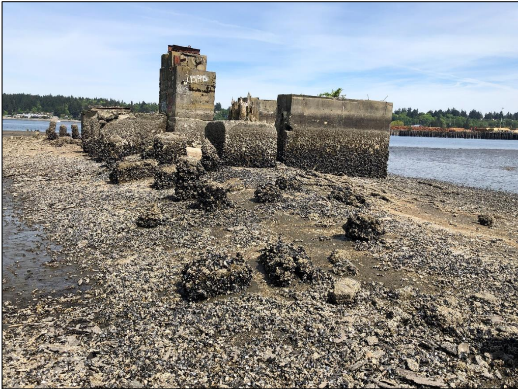
Photograph 6. Large concrete structures, debris and piling to be removed, located immediately waterward of property shoreline.
