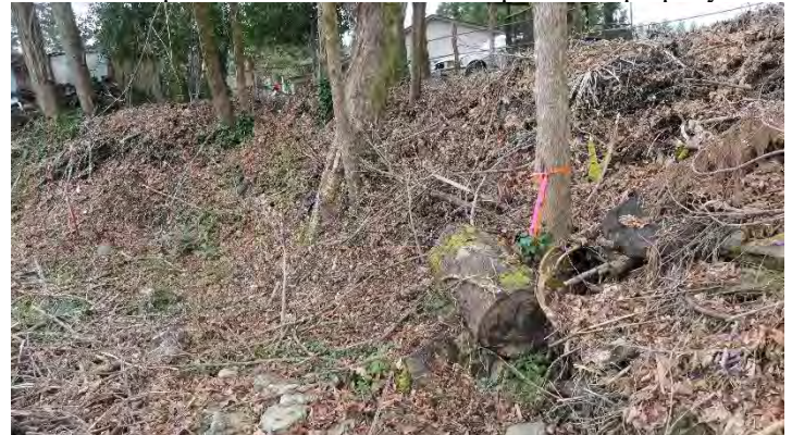
Photo 46. Cut slopes and cut trees in wetland buffer
