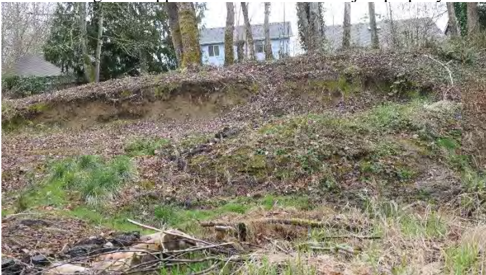
Photo 7. Cut material from slopes pushed into wetland
