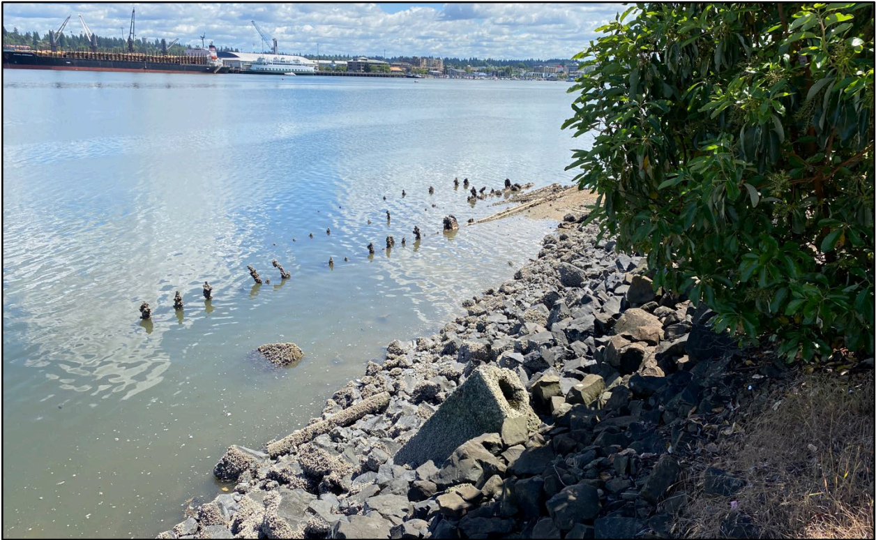
Figure 48. Overview of exposed piles from the floating platform east of the project site. View is southeast.
