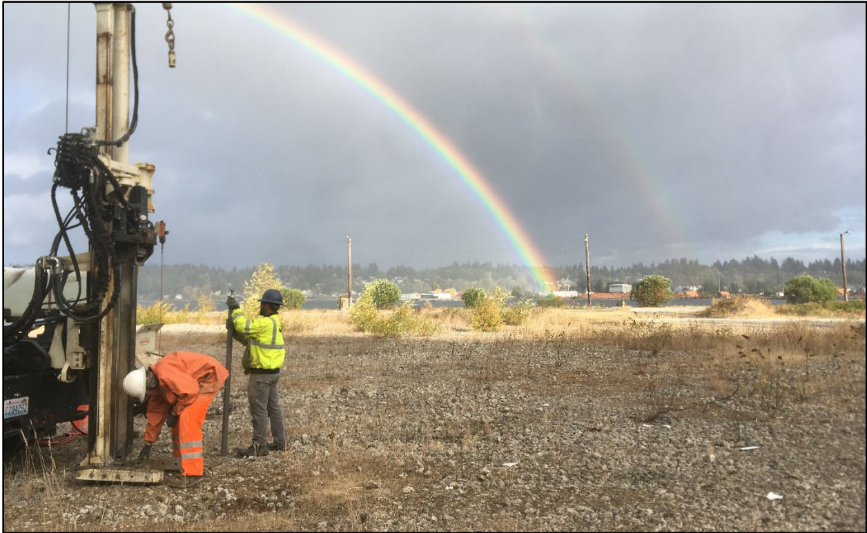
Figure 23. Overview of API with direct-push bore equipment facing east.
