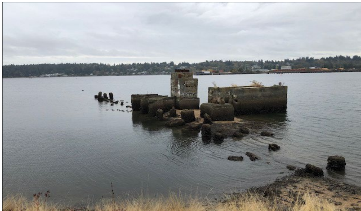
Figure 70. Overview of the piers and concrete platforms for traveling crane associated with the Northern Pacific Tumwater Branch Spurs (TSN: TH2022-1103), direction east.
